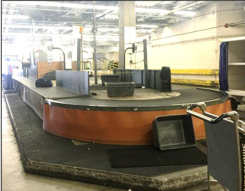
South Satellite Make-up Device
